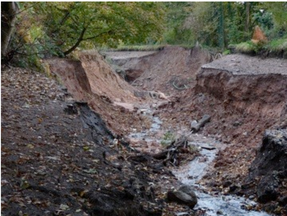
The devastated canal structure at Dutton Hollow on the T&M. Fencing and Fiber Optic cable conduits were left suspended between the remaining sections of tow path.
